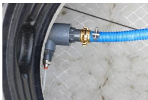
Fig-19 : Connection on the biological reactor side
