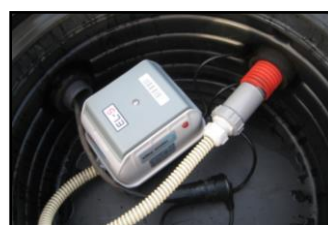
Fig-22: Electrical Connection inside a building
